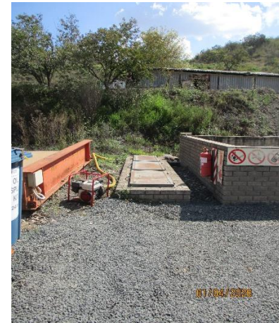
Photo 3: Oil separator attached to diesel tank bunding area.
