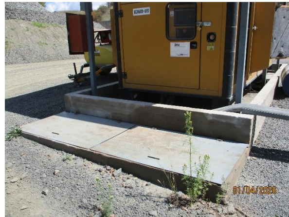
Photo 5: Generator in bund with oil separator attached (evident in the foreground of the photo).
