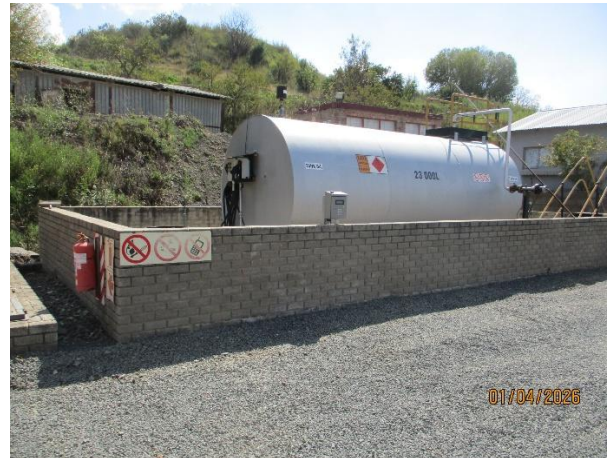
Photo 2: Above ground diesel tank and bund.
