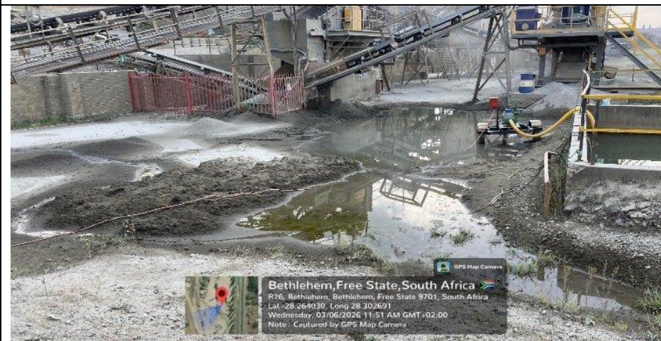
Photo C15: Work area requiring drainage channels.
